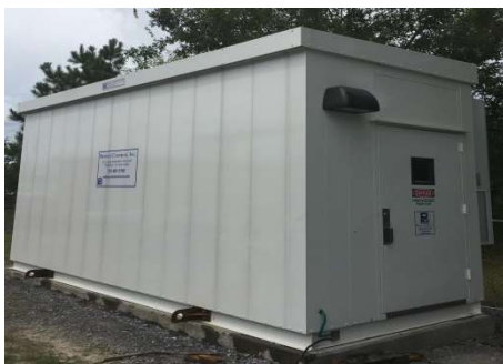
Custom Power Control Buildings
